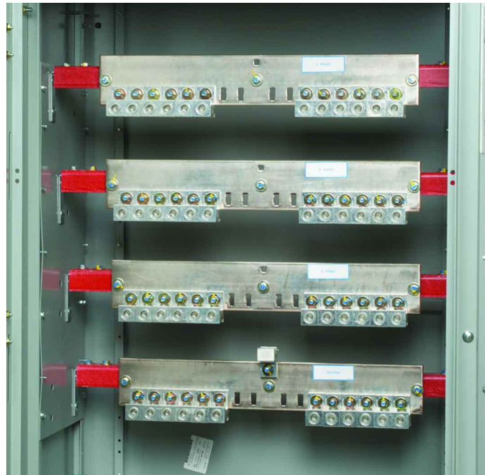
Mechanical Lug Terminations Shown
